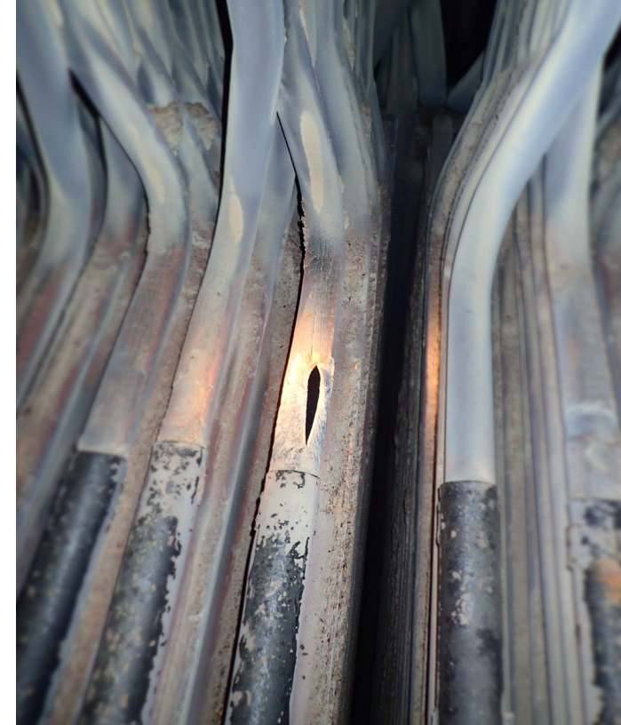
Reheat tube failures on NC2
